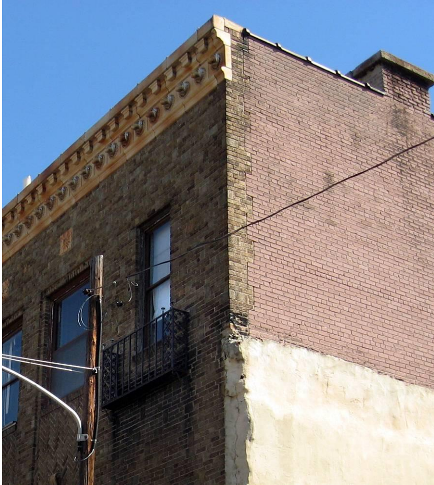
Figure 6P: Detail showing the exposed cornice profile, the manner in which the decorative facing brick wraps onto the south façade, the bracketed metal flashing, and the chimneystack.
