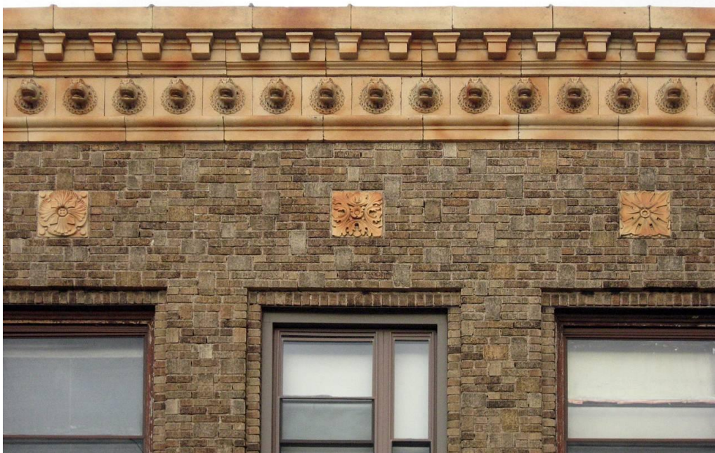
Figure 6I: The building's terra cotta cornice and the three different styles of terra cotta tiles found below the cornice along both the building's north and west façades
