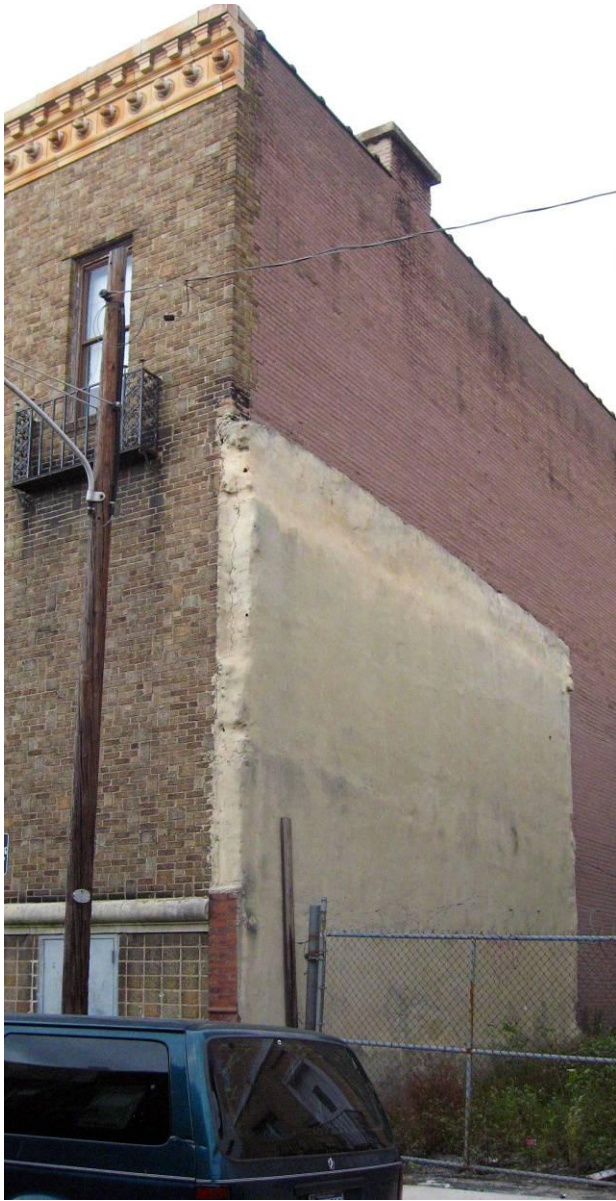
Figure 60: Exposed southern façade of the Stiffel Center. Image shows remains of the two-story rowhouse that was once adjoined to this façade.
