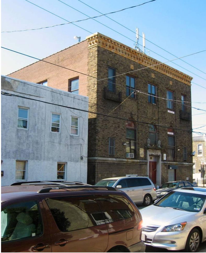
Figure 6L: Photograph taken from the northeast corner of Porter Street, at the intersection of Porter and South 6 th Streets. Looking southwest, the photo reveals how the decorative cornice and facing brick wrap onto the building's east elevation.
