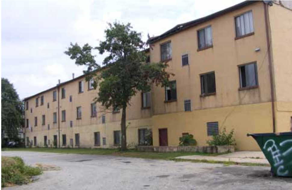
Left: Damaged roof and gutters contributes to water problems both inside and out. Signs of mold and mildew are evident along the exterior of the buildings.
